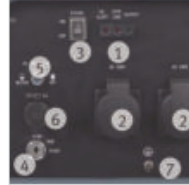
Panel de control PG-I 35 SE.
